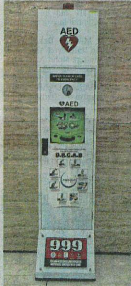
In case of emergency: An AED device installed at a hotel in Kuala Lumpur.
